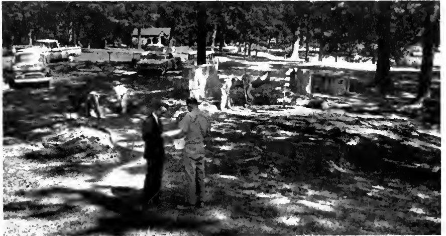
An on-site park maintenance workshop in Tilles Park, a St. Louis County facility, included construction of a complete children's playground during this popular session. (Photo by Bill Harris.)
