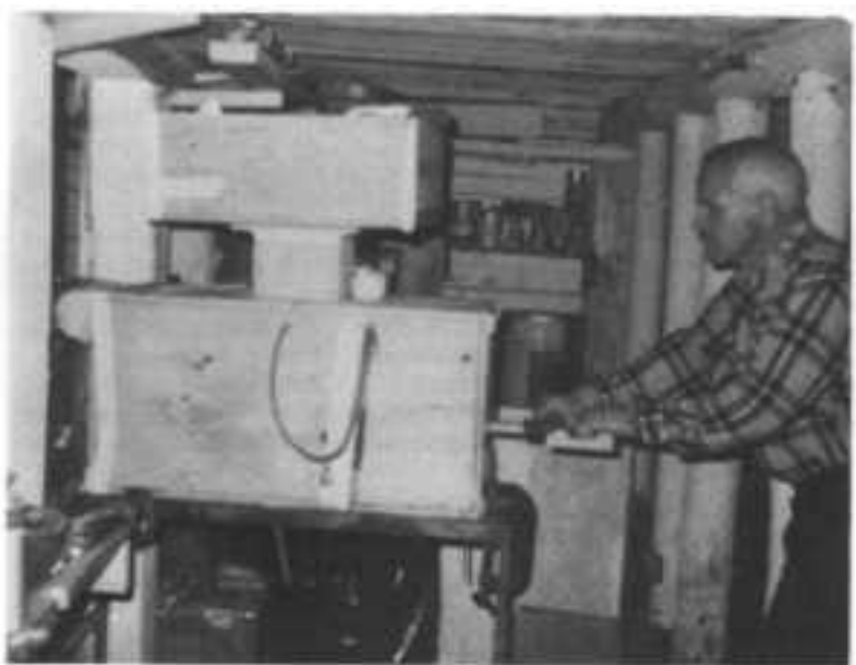
Fig. 3. Pump with Homemade Filter (20 x 20 x 8-inches inside dimensions) connected airtight on top of the pump's 6 x 6-inch air-intake duct.
