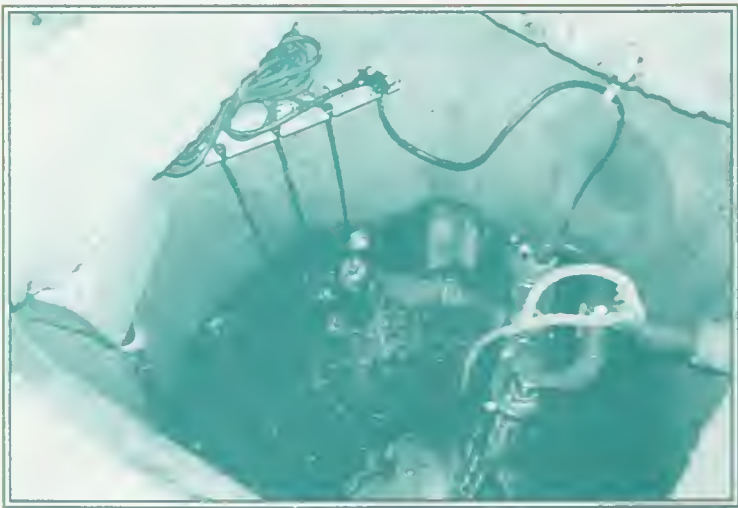
COMMUNITY, I.D. GAUTHIER STEP system: storage tank / pump chamber (see figure 16)
