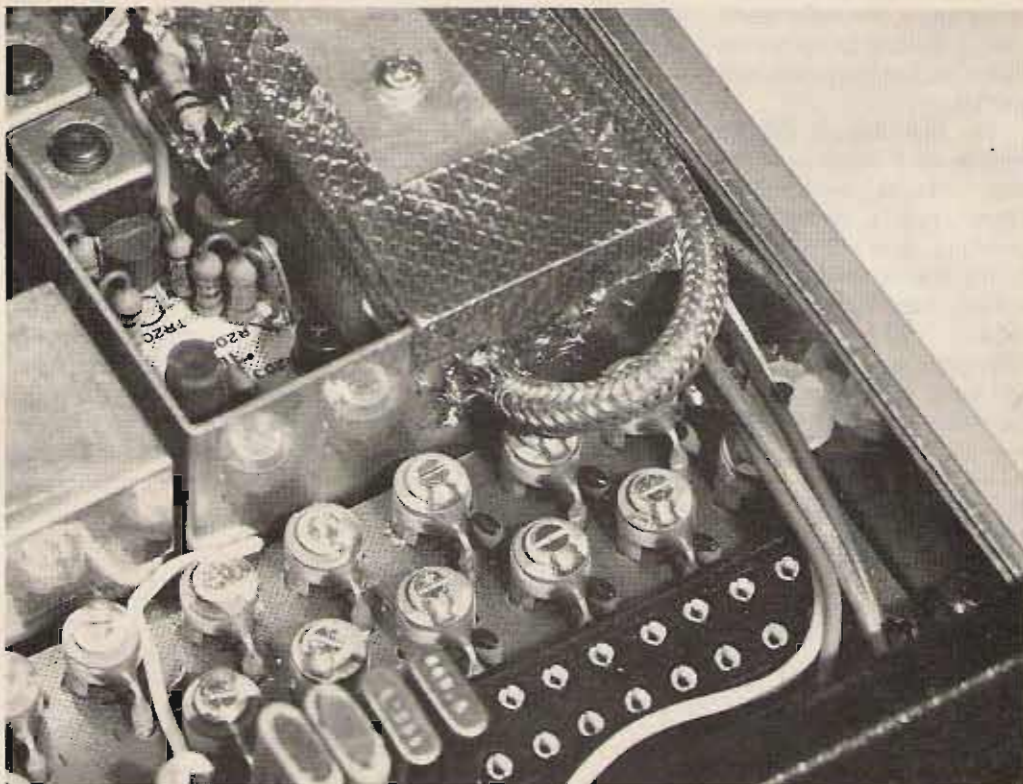
Front right view of the transceiver with the top cover removed, showing the receive coax cable entry into the rf compartment. Note that the outer braid is soldered to the outer wall of the compartment.
