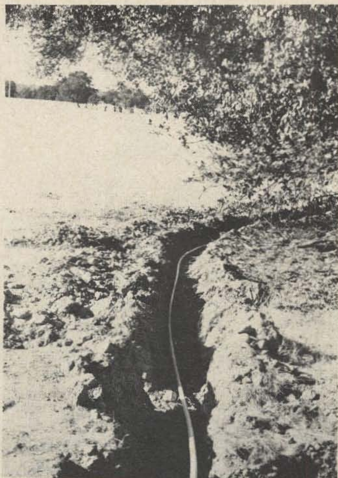
Plastic pipe in trench containing feed coax and antenna switch wire.
