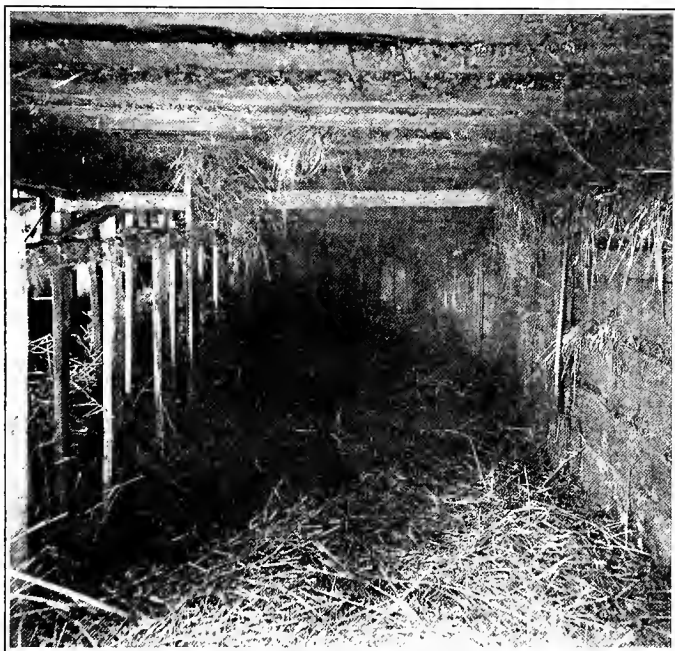
FIG. 9. — An old barn with cracks filled with straw is not a sanitary place in which to milk.
