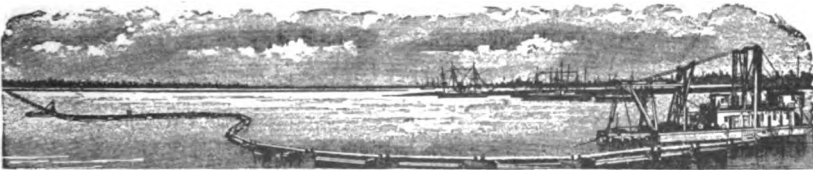
Hydraulic Dredge discharging through 5,700 ft. Pipe. Will dig and put ashore any Material, Rock excepted.
