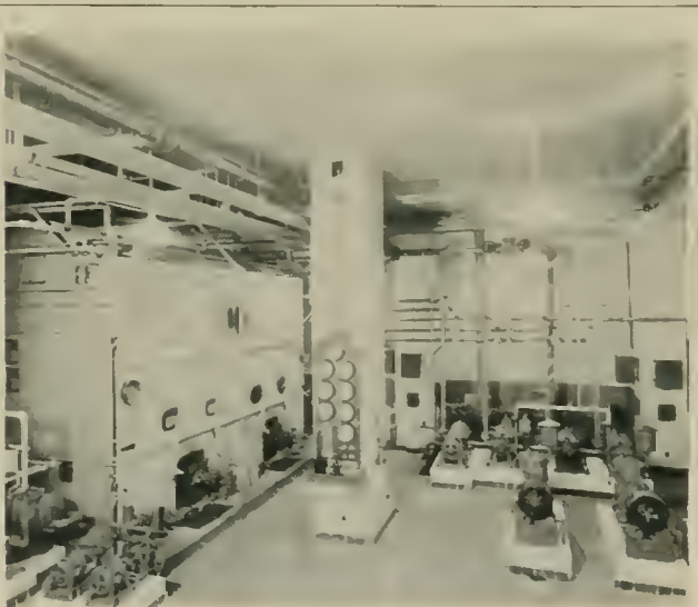
SUB-BASEMENT INSTALLATION, COAST DIVISION BUILDING P. T. & T. CO., SAN FRANCISCO
