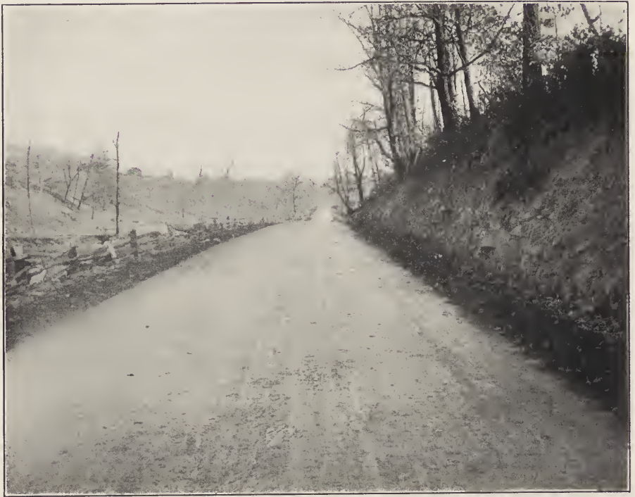
CONCRETE ROAD, GARRET CO., MARYLAND 10% Addition of Hydrated Lime to 1-2-4 Concrete (Monolithic Type)
