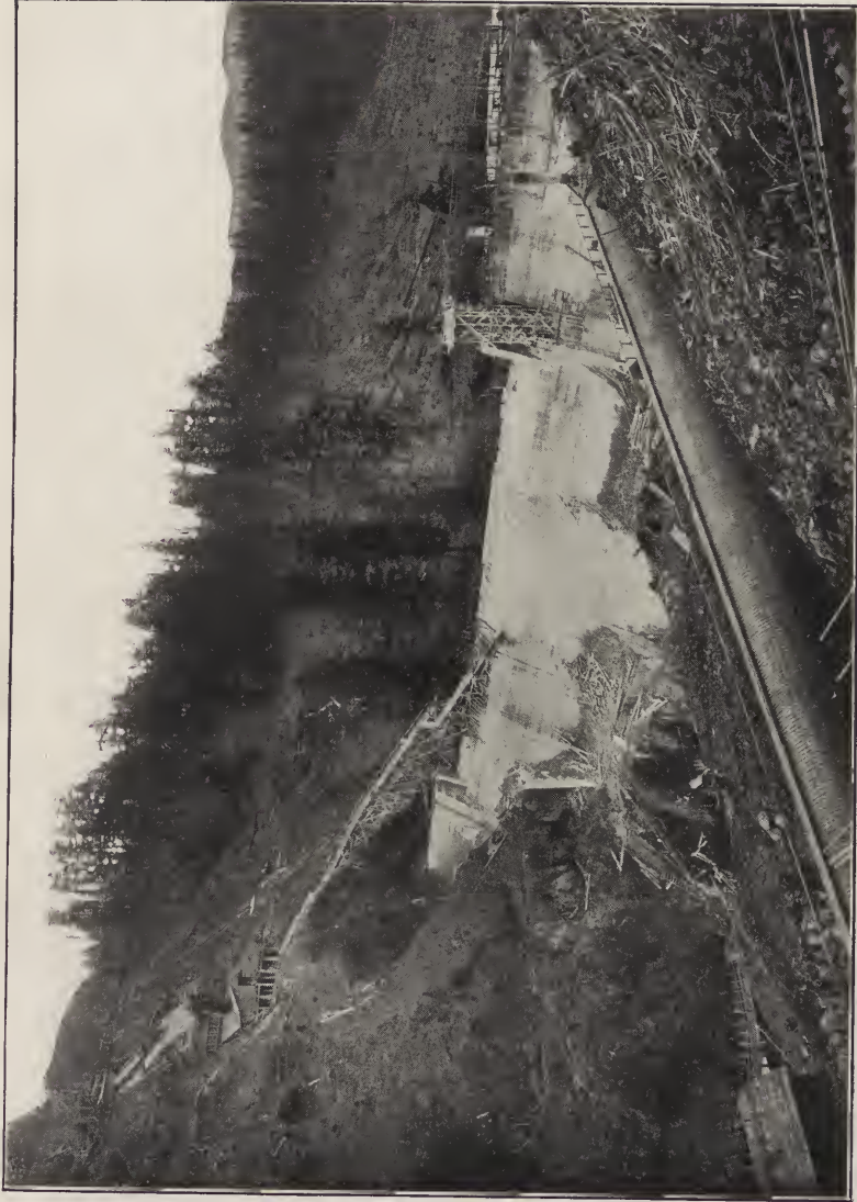
DAM, WHITE SALMON RIVER, WASHINGTON (UNDER CONSTRUCTION) 10% Hydrated Lime Used in All Concrete
