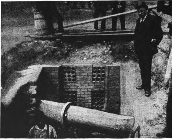
Fig. 50. Manhole, Market and Washington Streets, Chicago.
