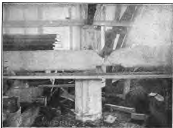
CUT SHOWING FAILURE OF BEAM NO. 1.
