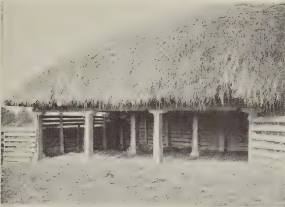
Concrete footings and concrete posts provide strong, durable supports for this cattle shed. They will not decay.
