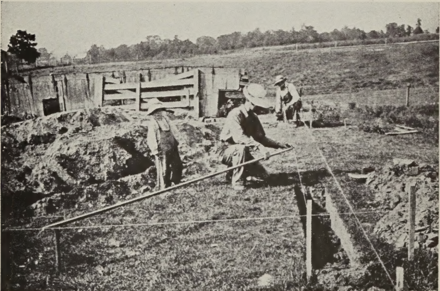
In the absence of surveying instruments a corner may be tested for squareness by the simple method shown in this illustration. Definite instructions for laying out a foundation are given above.
