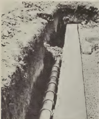
A line of concrete drain tile placed on the outside of the footing assures a dry basement.
