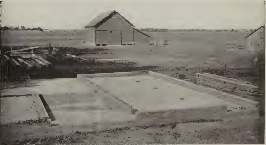
Concrete foundation and floor for a corn crib and granary. Bolts have been embedded in concrete for the attachment of sills.
