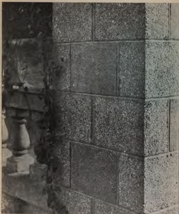
FIG. 61—DETAIL OF CONCRETE BLOCK HOUSE WITH TWO GRADES OF FACING, BRUSHED WHILE GREEN—R. H. BUSHNELL
