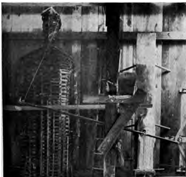
FIG. 42—BUILDING FRAMEWORK FOR CLAY MODEL 16' HIGH FOR CONCRETE STATUES, USING PANTOGRAPH IN CONNECTION WITH \frac{1}{4} -SIZE MODEL
