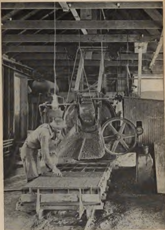
FIG. 15—GANG MOLD FOR 20 BLOCK, MOUNTED ON TRUCKS BEING FILLED WITH SLUSH CONCRETE DIRECT FROM MIXER CHUTE
