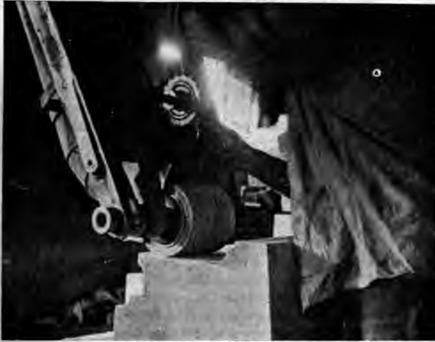
FIG. 80—MACHINE FOR FINISHING CONCRETE IN PARALLEL CUTS OF FROM \frac{1}{8} " TO \frac{1}{4} " WIDE
