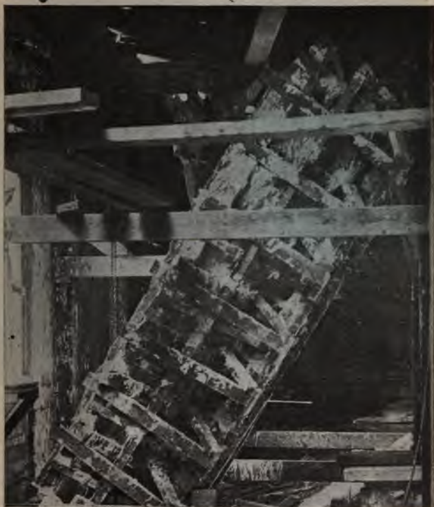
FIG. 45—TURNING CRADLE CONTAINING PLASTER MOLD FROM VERTICAL TO HORIZONTAL POSITION FOR FILLING WITH CONCRETE
