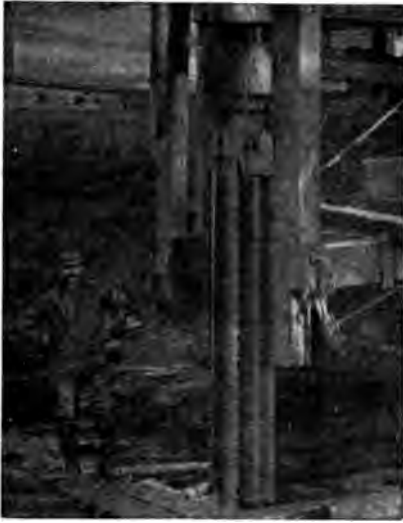
Driving a Section of Wemlinger Piling. Note total absence of buckling, although the pile extends about 12 ft. into the hard ground.
