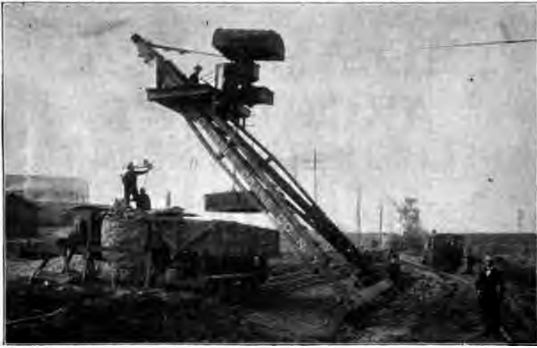
The photograph shows one of six Balanced Cable Cranes at work on the Erie R. R. cut, Bergen Hill, Jersey City, N. J.
